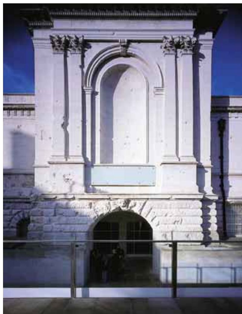
Una porta, aperta in quello che era un basamento cieco (a sinistra), conduce al nuovo salone d'ingresso (a lato) A door pierced through what was a blank basement wall, left, opens into the newly created entrance hall, facing page
